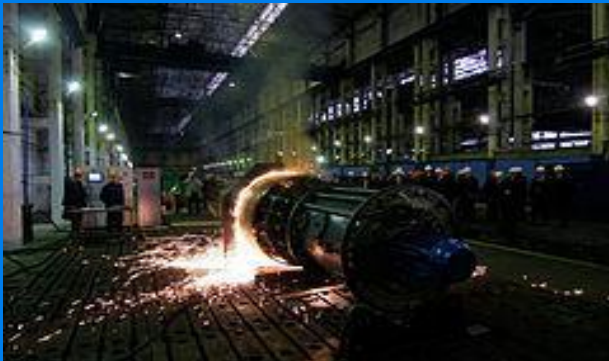
Contact welding by continuous reflow of a gas pipeline with a diameter of 1420 mm in Pskov at the TPP0 plant
