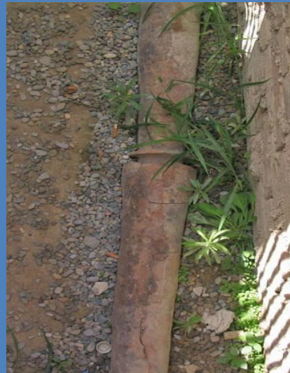
for waste water
