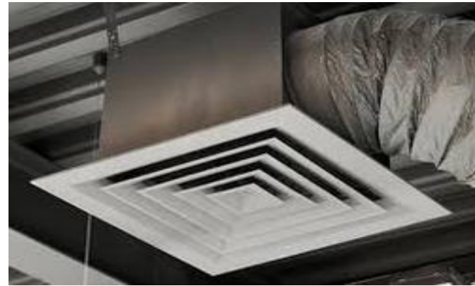
Centralised Air Conditioning
