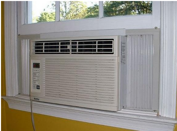
Window Air Conditioning
