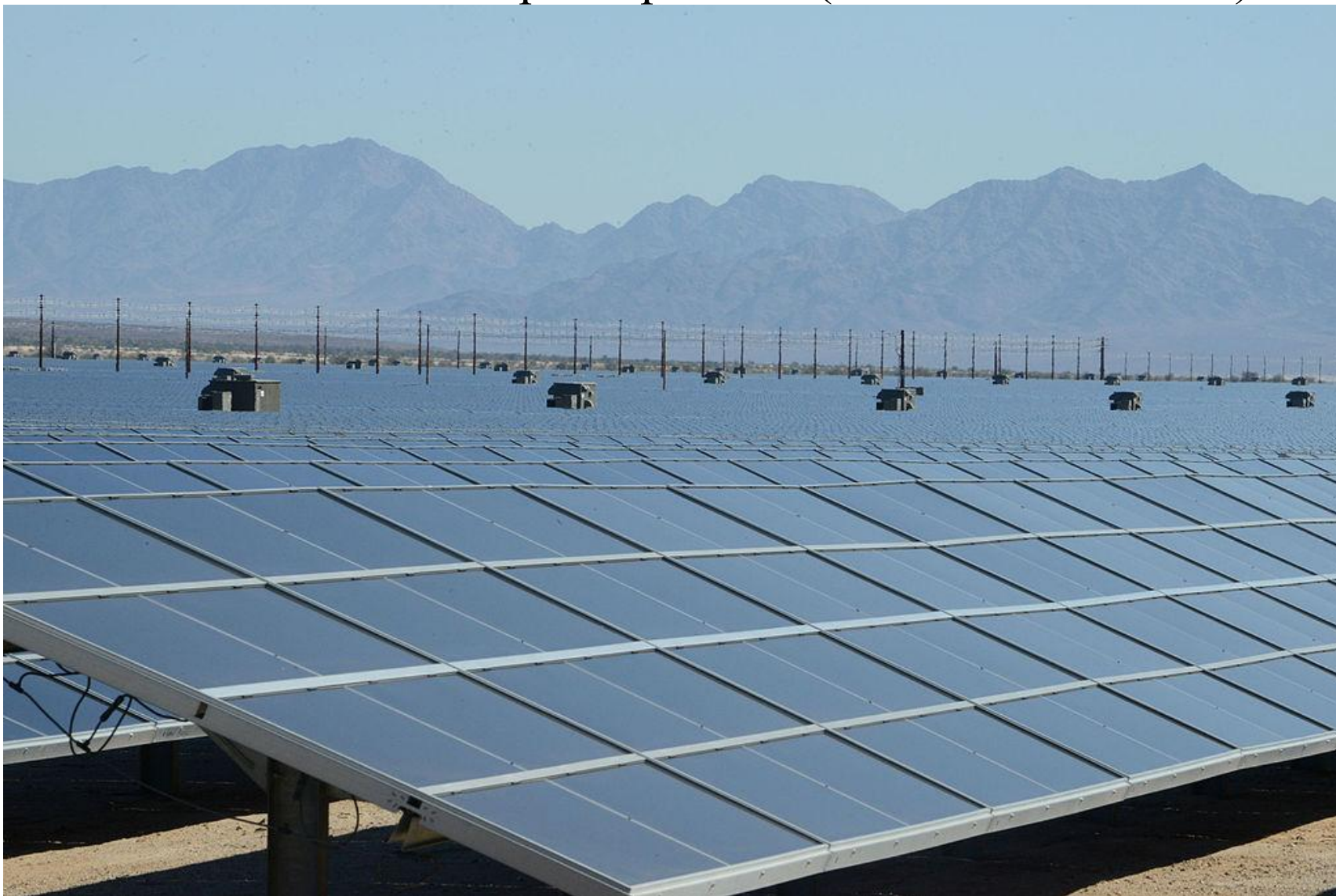
The 550 MW Desert Sunlight Solar Farm
