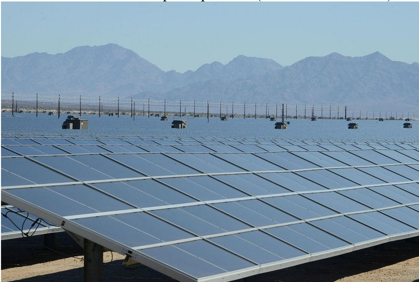
The 550 MW Desert Sunlight Solar Farm
