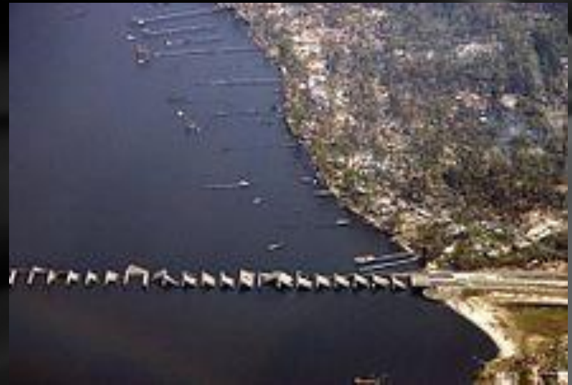
U.S. Route 90's Bay St. Louis Bridge on Pass Christian was destroyed as a result of Katrina.
