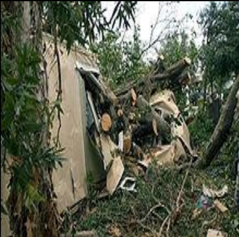
Damage to a mobile home in Davie, Florida following Hurricane Katrina
